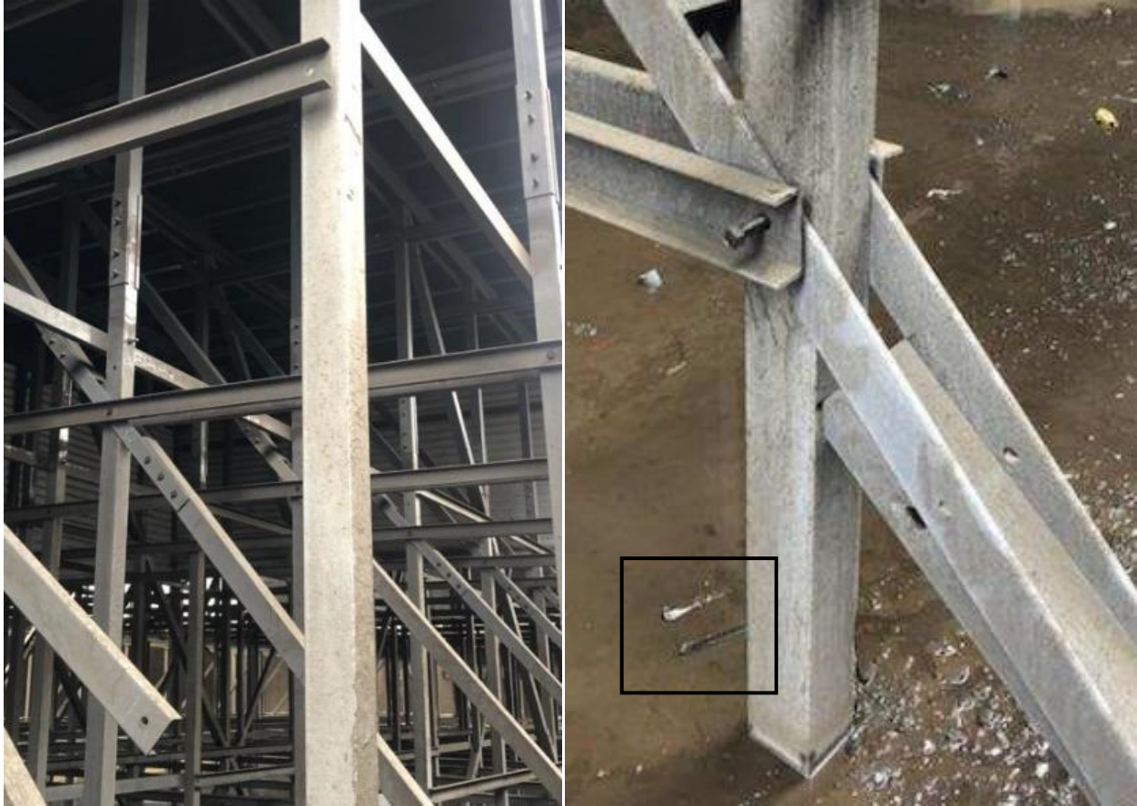
FIGURE 2 LOOSE AND MISSING BOLTS FOUND DURING SITE INSPECTION
