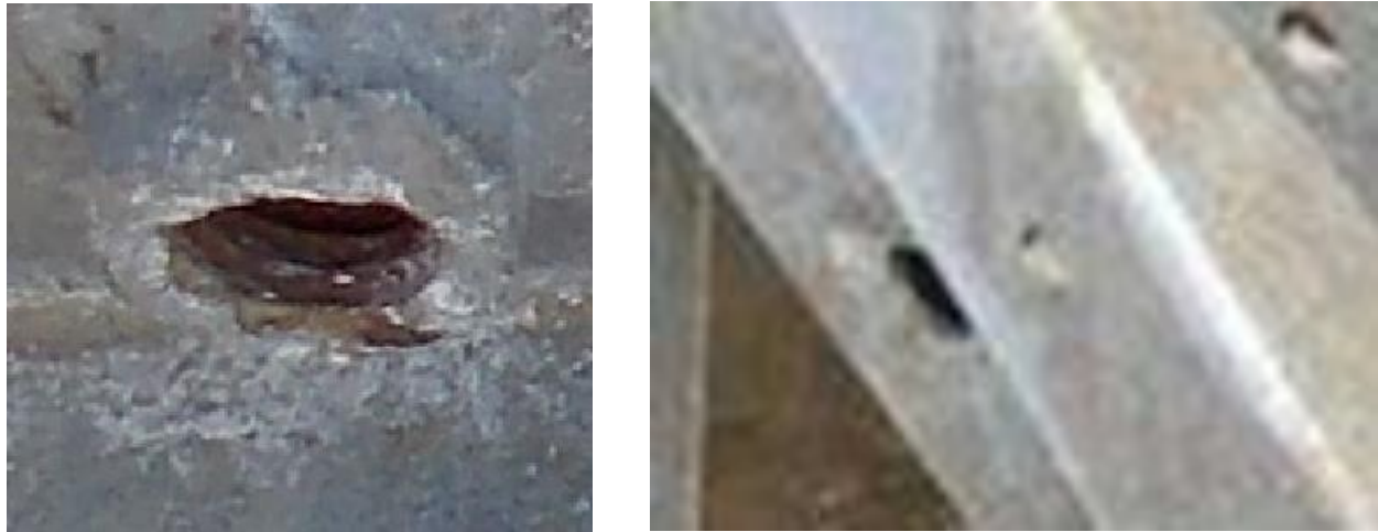
FIGURE 3 DAMAGED BOLT HOLES OF PINNED CONNECTIONS
